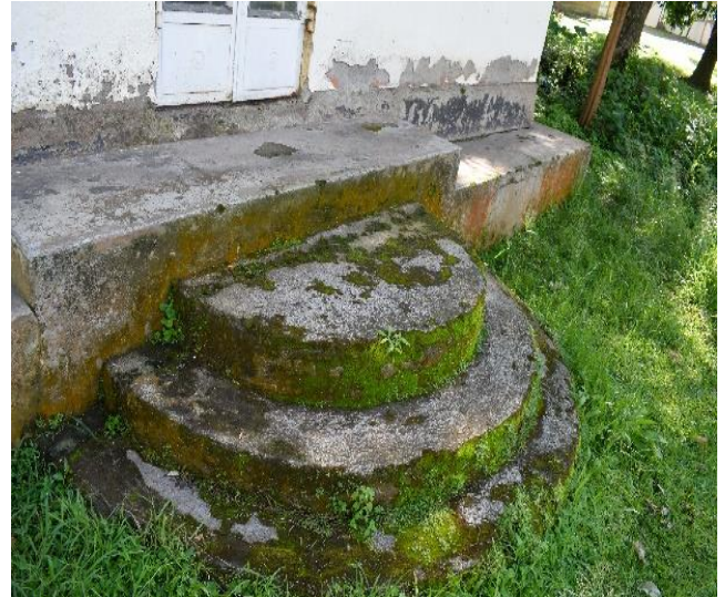
Algae infested damaged stairs at Itwara sector Office
